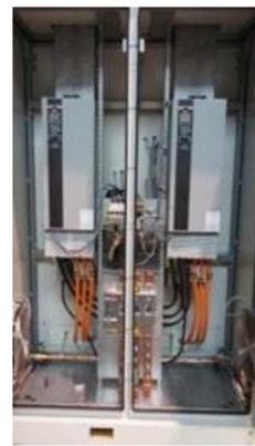
Compressor drives + main power connection
